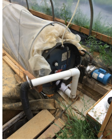
Figure 5. Discharge of effluent (PVC tube) and recycle pump (right)
