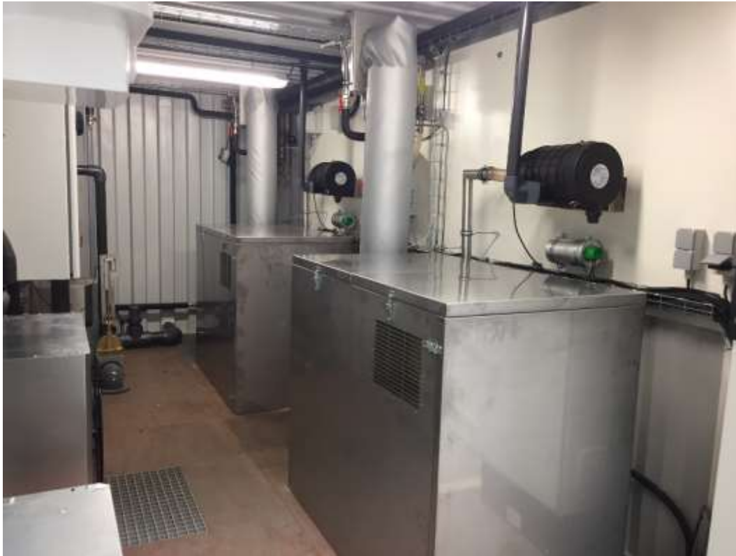
Inside the mini-digester power/control container. Two Kubota CHP units in noise dampening enclosures, with exhaust heat recovery shown. Photo by Martin Energy Group
