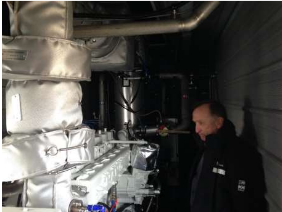
Lee Lutz with 150 kW CHP genset at Kurtz Valley Holsteins, built by Martin Energy Group. Note the flexible insulation around exhaust gas heat exchangers. Manure from the farm's 330 mature milk cows will be mixed with food waste to produce gas to power the engine.
